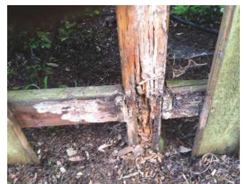
A rotting fence post
