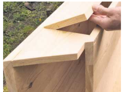
13 Cut the door to size, bevelling the leading edge so it doesn't bind against the front panel
