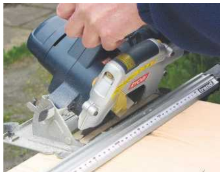
6 Tilt the saw blade over to 30° and cut the top edges of both front and rear panels
