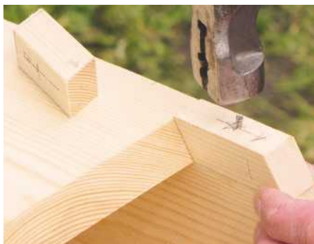
14 Add angled blocks at each end of the letter opening to extend the sides. Glue and join
