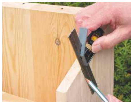
16 Biscuits help locate the roof in position, though it's best to add screws as well for security purposes
