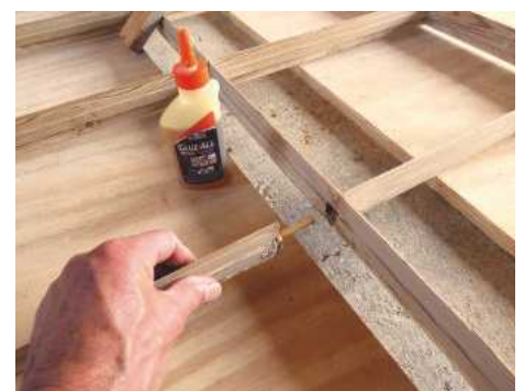
24 During dismantling it's likely that one or two existing pins will snap off. Where necessary, drill out bars to accept new dowels
