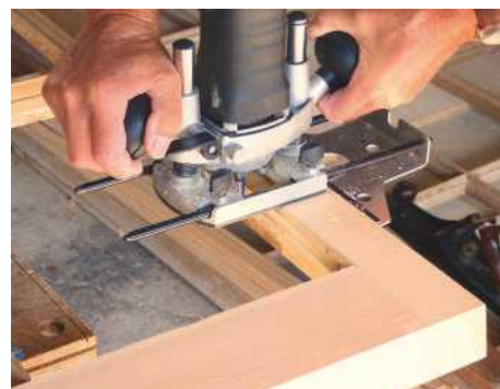
30 Tidy up the inner rebates of each new stile with a router, where necessary. Trim the internal corners square with a sharp chisel
