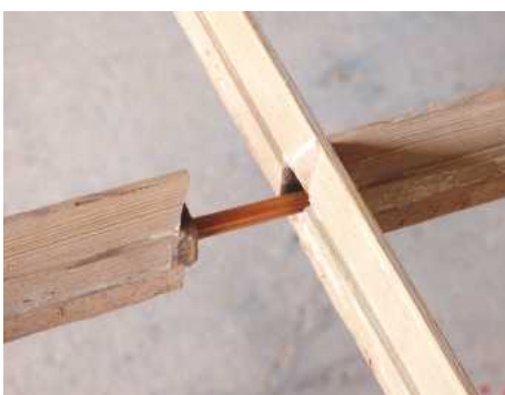
22 Each vertical glazing bar intersects with its adjacent horizontal bar via a hardwood pin, set into a matching mortise
