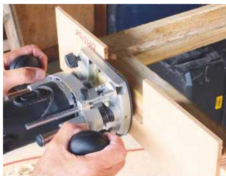
32 When several hinges need to be fitted it's easier to make an MDF jig for the housings. Cramp to the top rail, then rout the recesses
