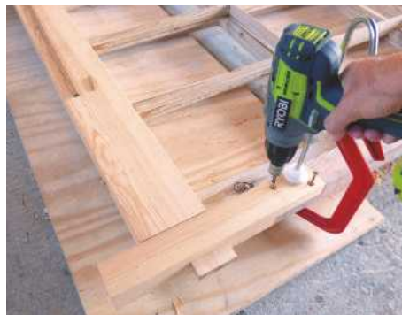
17 Dry assemble the corner joints. Drill clearance holes, align the new stiles with the original sash and screw them together temporarily
