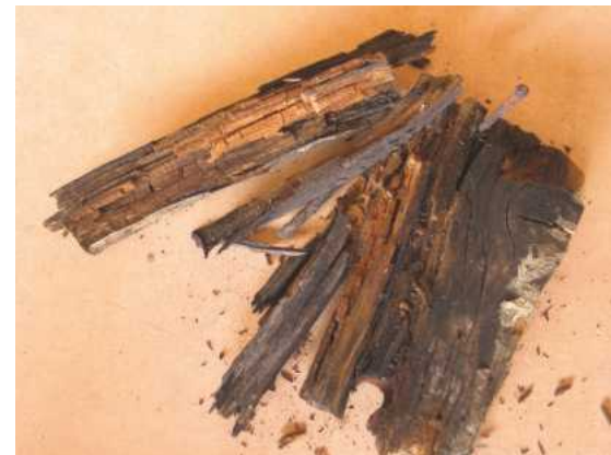
Friable and longitudinal damage caused by wet rot
