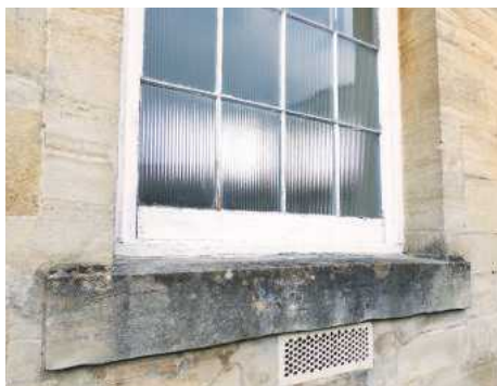
1 Each window had two lower rows of reeded glass. Putty was loose or missing and paintwork was generally in poor condition
