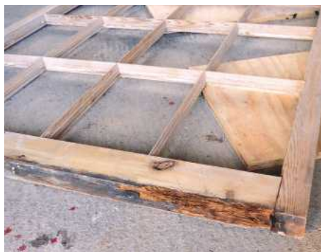
2 After removing each fixed sash from its frame all glass was taken out. All windows were then stripped chemically to remove paint
