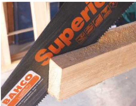
16 Saw off the ends of the stiles on the original sash. Mark out at the same gauge setting and clean up surfaces as necessary
