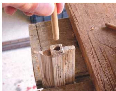
23 Where existing pins have snapped off, replace with hardwood dowels. Glue in place and cut to size, about 50mm protruding
