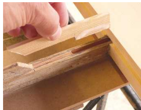
27 As these glazing bars are so slim they split easily. Repairing them means narrow chisels, sharp planes and light cramps
