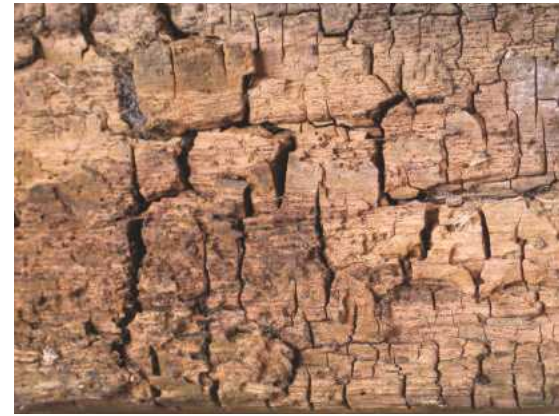
Typical cube-like damage caused by dry rot
