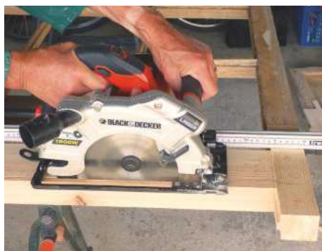
29 Saw off the excess horns. Mark the sash for length, then cut a bevel along the lower edge of the bottom rail with a circular saw
