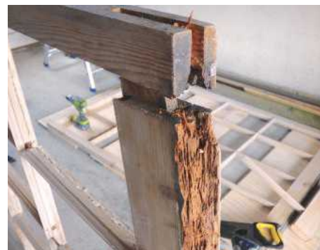
3 You need to assess work carefully before starting a project such as this. All the lower mortise & tenon joints had rotted badly
