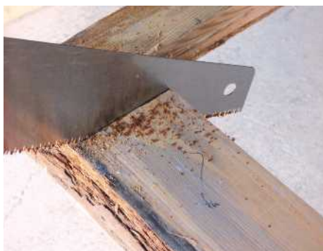
4 Support the sash off the floor and saw through the bottom rail at each end
