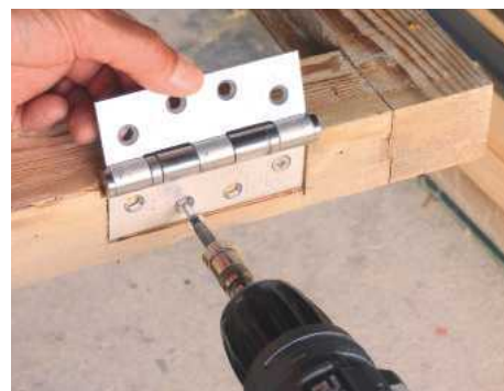
33 Drill and fix the hinges in place using stainless steel screws. Mark and cut the matching recesses in the head of the frame
