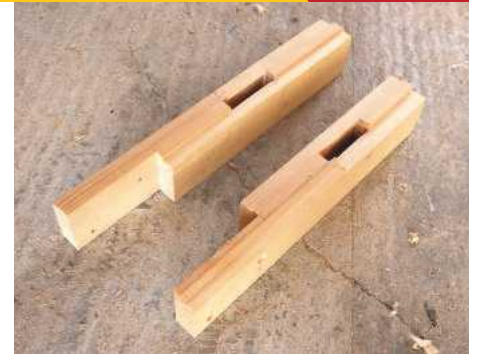
15 Using a marking gauge, mark a halving joint at the end of each new stile. Cut away waste and clean up with a shoulder plane
