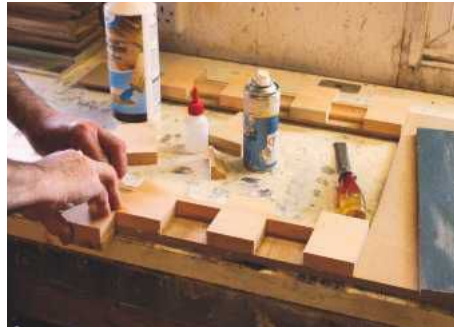
5 Architrave being glued in place with the aid of a spacing 'gizmo'
