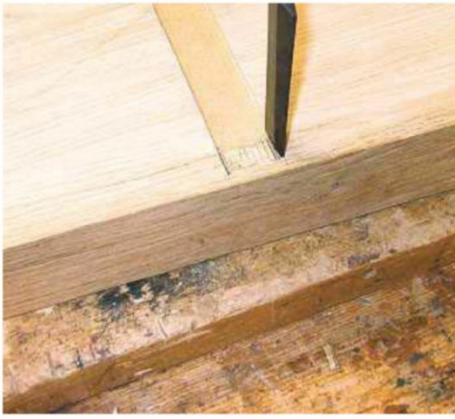
9 Use a sharp chisel to clean up the stopped housings after the lippings have cured
