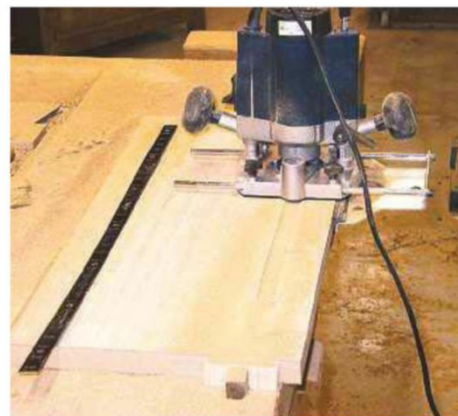
3 Rout housings for the shelf tracking; a dedicated cutter will rout the deeper central recess for the studs at the same time
