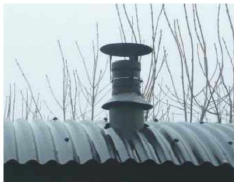
A lead slate is provided for the chimney
