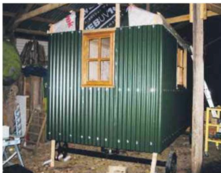
The corrugated cladding is now fitted and allows a 25mm air gap to the breathable membrane and insulation within
