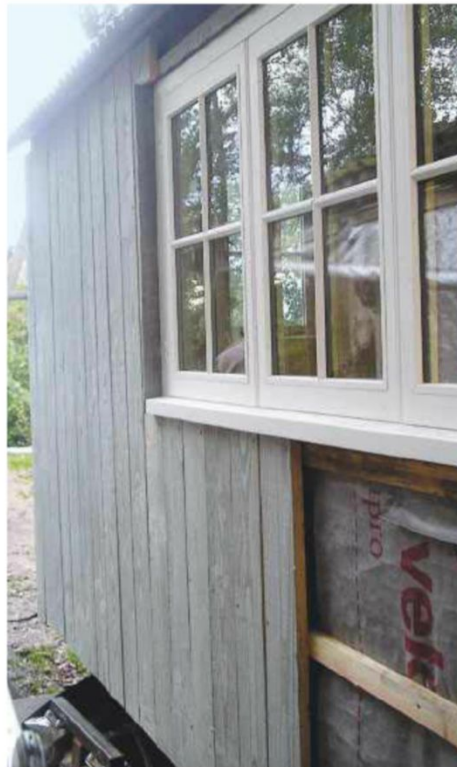
50mm of wool insulation between the frame members outside of the plywood, which is then covered with a breathable membrane
