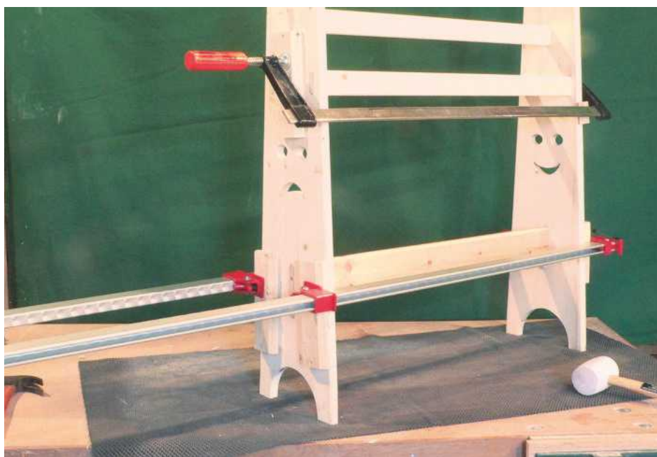
12 Three sash cramps held the structure together overnight while the glue went off
