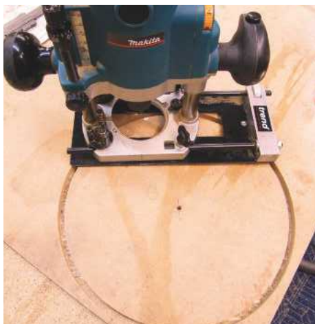
3 Pin the MDF onto some scrap to prevent the cutter kicking the side as it breaks through
