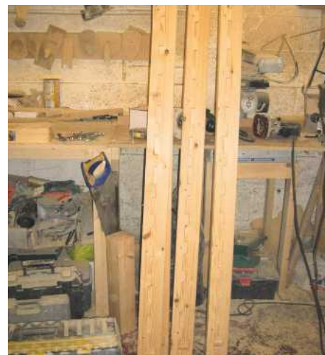
17 Bearers were attached to the insides of the rails with glue and screws
