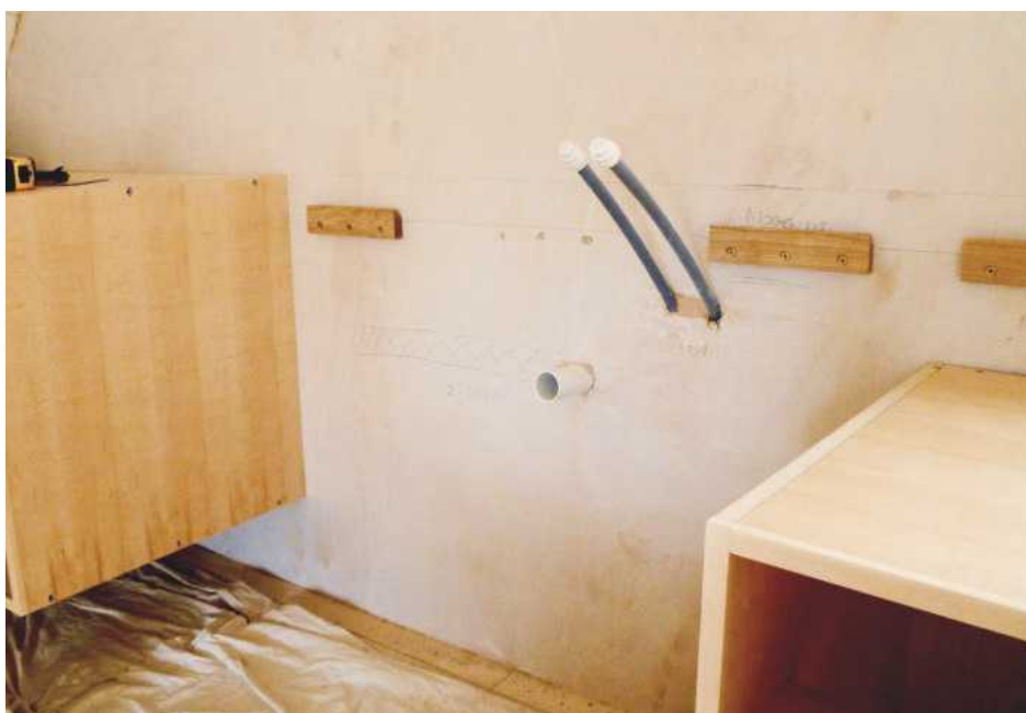
10 Pipework and French cleats on the wall
