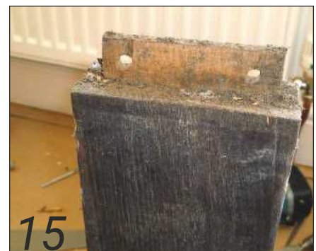
Break-out around left hole that needs attention
