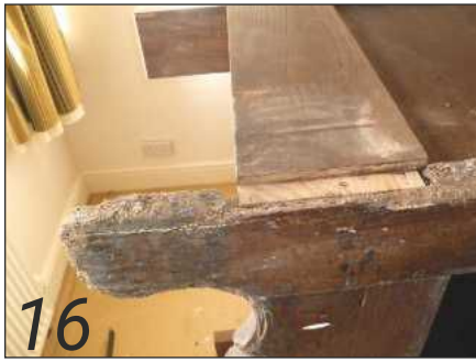
16 Damaged area on front stile requires repair
