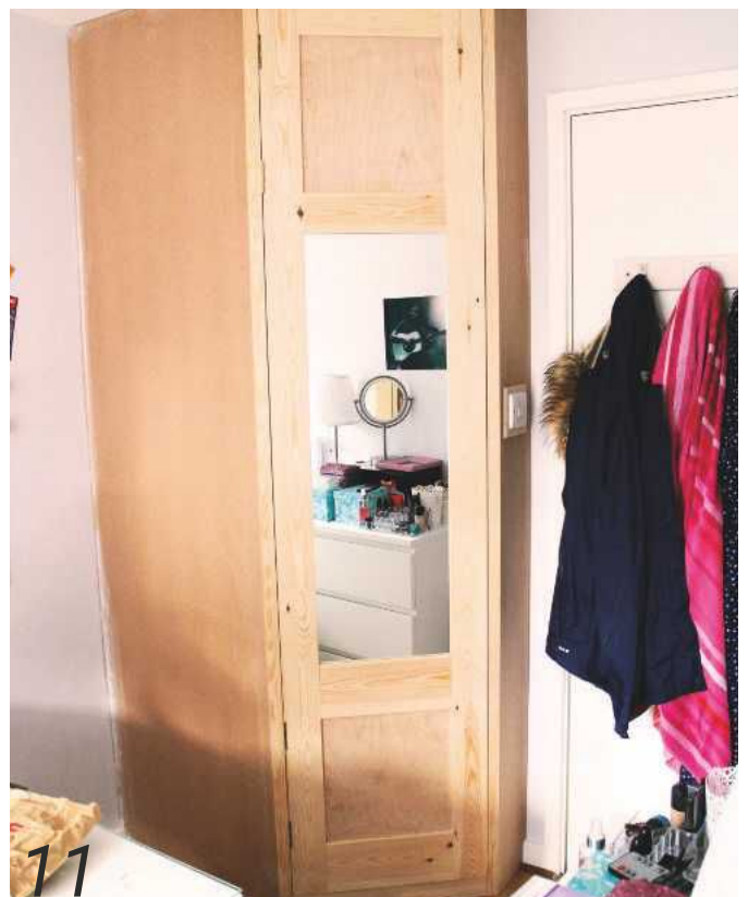
11 The (almost) finished job; it should almost disappear into the corner when it's painted to match in
