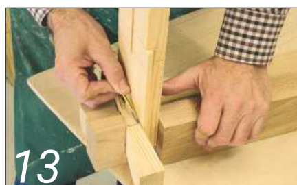
13 A wedge is used to mark the angle for the outside edge of the trench, which is cut by hand saw
