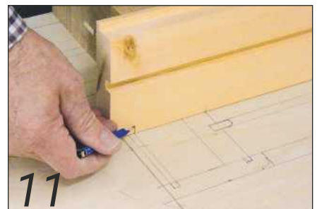
11 The head is marked for trenching out by lifting the sizes directly from the rod
