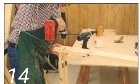
14 The head, sill, and pulley stiles can now be assembled and placed to one side
