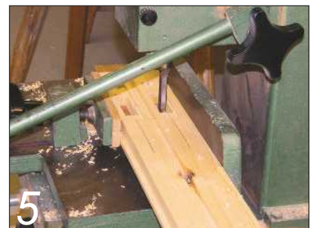
5 A combination of router and mortising machine forms the recesses for the pulley wheels
