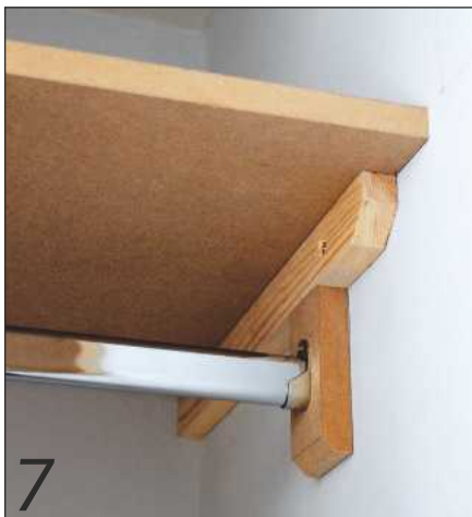
7 While access is at its best, fit any shelving and rails. Note wall block to assist the rail bracket fitting
