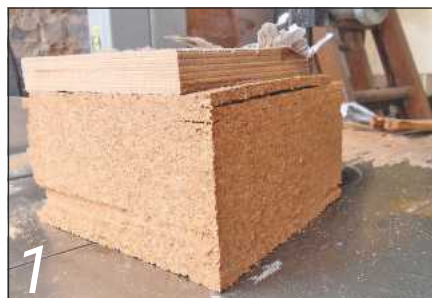
1 Laminate the cork tiles and layer them up until they are approximately 90mm-thick
