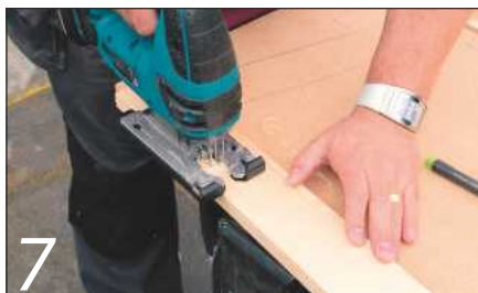
7 This is then cut with a jigsaw and used as a template for the opposite piece
