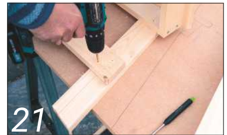
21 You can then screw the rails in position to the inside of the legs
