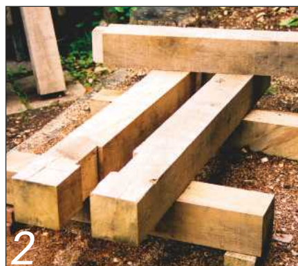
2 Lay the two stabilisers roughly parallel, 1m apart, and lay the lower beams on top
