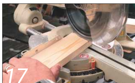
17 Cut to length on the mitre saw. A laser comes in handy here for accurate working
