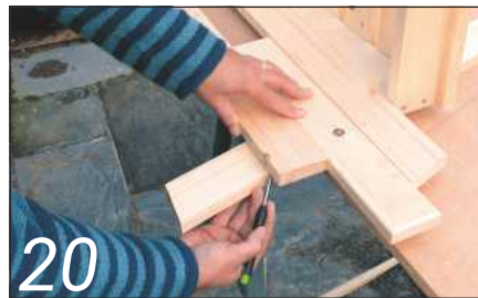
20 Side rails are spaced and positioned directly to the legs and marked for cutting
