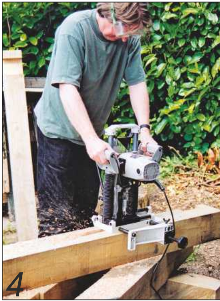
4 I used a chain mortiser to cut out the long channels in each upright post...
