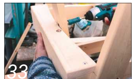
33 Fix the slat centrally to the seat back with the same sized screw
