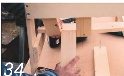
34 Use an offcut as a spacer to set the outer back rails
