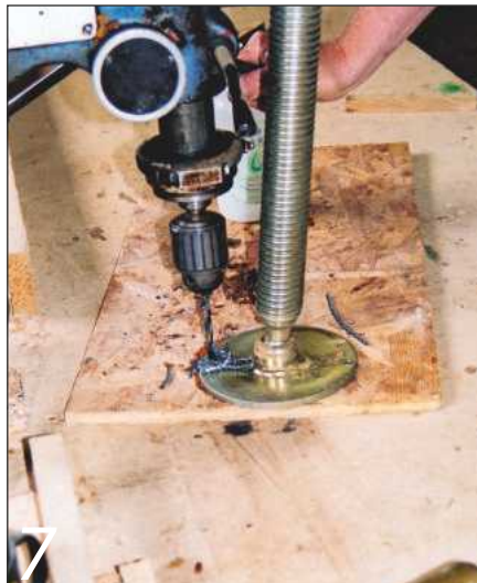
7 Drill and fix the lower beams to the posts with M10 threaded bars
