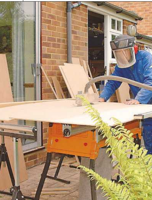
You can cut MDF into strips to use for skirting easily and efficiently with a table saw
