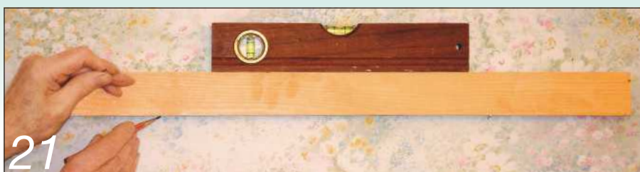
21 Supported by a temporary pin, the positions of the holes are marked out
