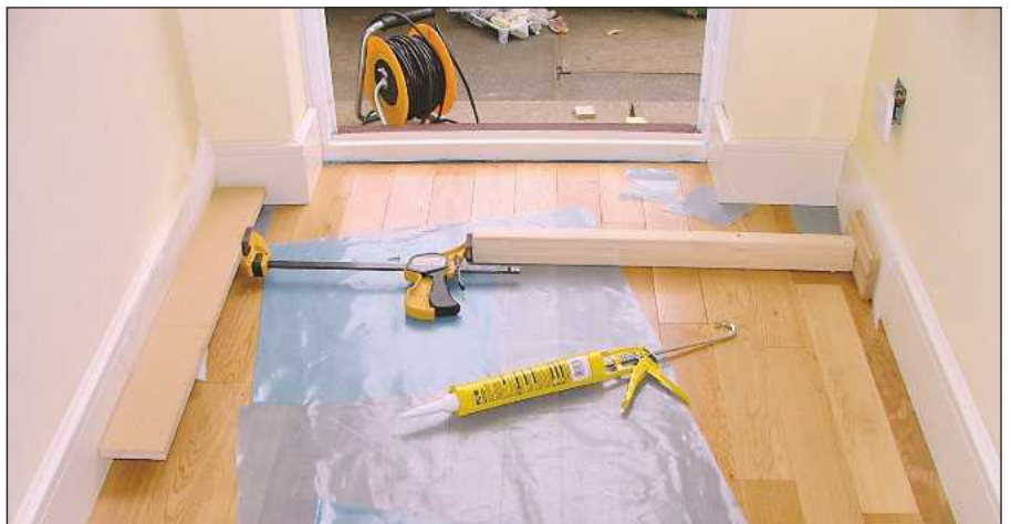
Clamps and a piece of timber can be used to hold the skirting in place
