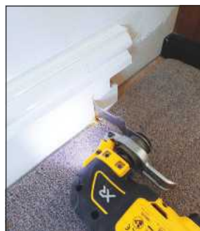
Using the Nail Buster blade allows plunging cuts through into the plaster below
