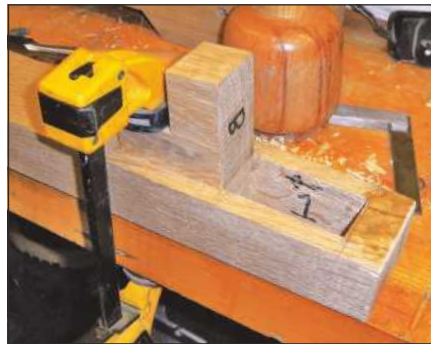
The tapers in the upper cross-brace mortises were cut with the help of an angled guide...
