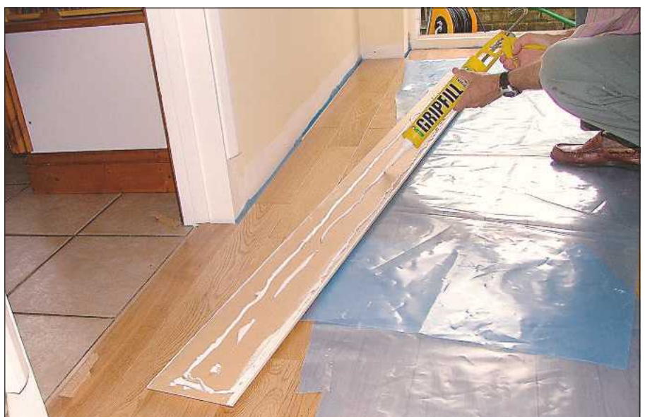
Apply gap-filling adhesive to the rear of each length of skirting in turn and press them into position
