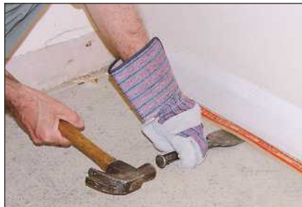
Use a bolster chisel and hammer to prise old skirting, floor coverings and gripper rods
