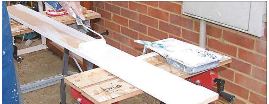
When all the lengths are cut to size, apply primer, undercoat and the required finish
