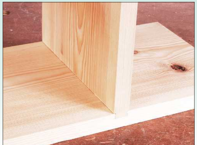
12 The finished joint. It should be a tight fit and may need tapping home with a hammer and a woodblock
