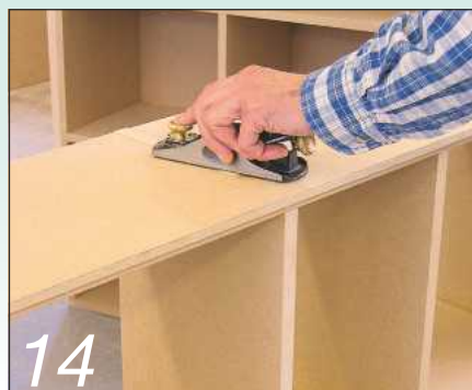
14 ...and a small block plane to clean up the protruding shelf ends
