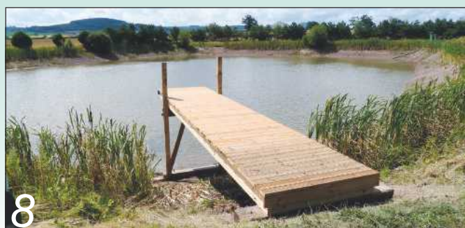
8 A few hours later the job was finished, and it made a very impressive addition to the surroundings. All we needed now was some rain...
