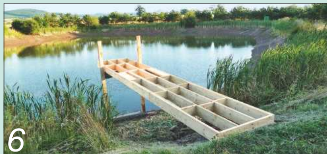
6 Getting the deck level and secure on its support frame using an array of levers and blocks took us most of the second morning
