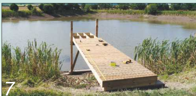
7 We started fixing the decking boards to the frame, but by lunchtime we had to take a short siesta because of the intense heat!
