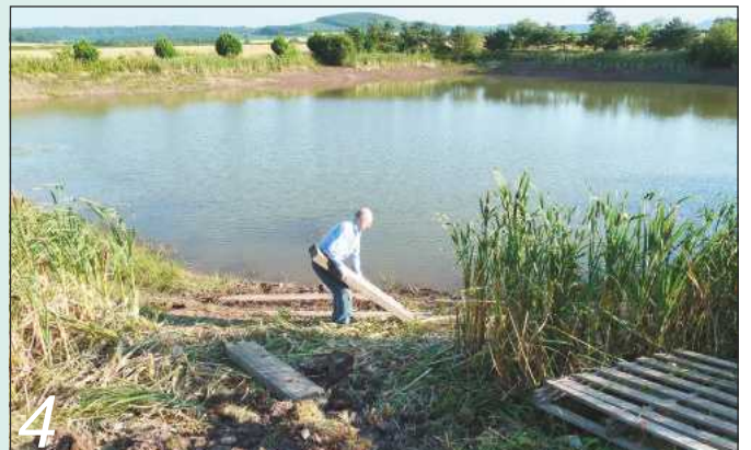
4 Despite the heat the bank was quite muddy, which made moving the heavy oak beams into position something of a challenge
