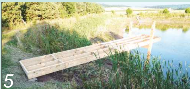
5 We eventually managed to manhandle the deck frame roughly into position on its supports... and then headed home exhausted by our exertions
