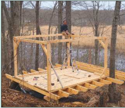
Existing trees lent support to the base, which was designed to allow for their future growth
