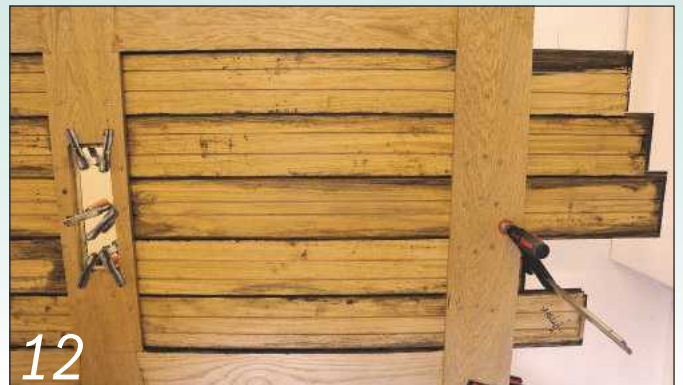
12 Fit and cramp the lower boards and screw them in place from the back
