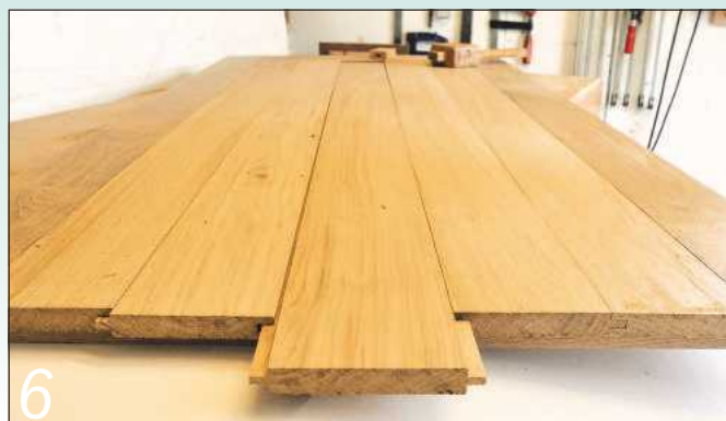
6 Cut the outer boards to length. The centre board is tongued on both edges
