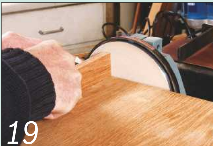
19 Prepare the shelf, then glue it and screw it in place from the back and sand its ends flush
