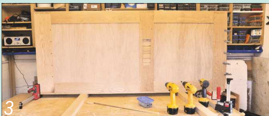
3 I cramped the door on edge and screwed the boards in place from the back
