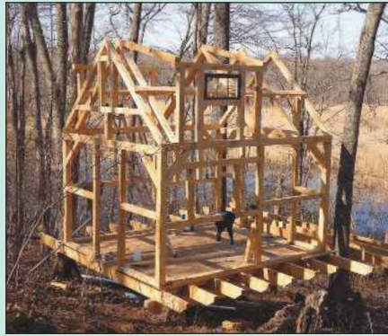
With the base completed, the house structure soon began to take shape
