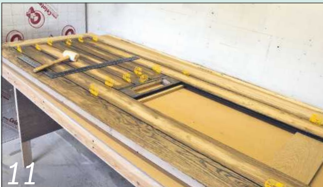
11 Dismantle the door, stain all the edges and begin the final assembly
