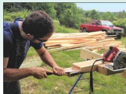
Dave quickly learnt to form bare-faced tenons with a Skilsaw and a large chisel
