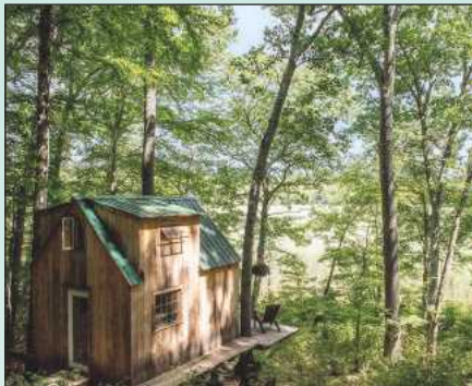
With the roof on and doors and windows in, the Wee House was almost complete
