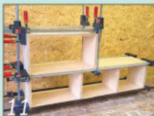
11 ...and helps to ensure that all the components come together perfectly square
