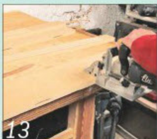
13 Cut slots for biscuits in the edges of the side panels and the backs of the columns
