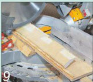
9 ...and to cut away the waste on alternate sections with a series of overlapping cuts
