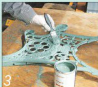
3 Use a small brush to apply two generous coats of special paint for outdoor metalwork
