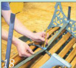
18 Bend the diagonal brace to shape and mark the position of its centre fixing
