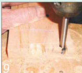
9 Bore out the bulk of the waste and remove the rest by chiselling
