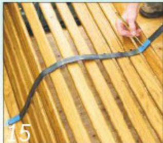
15 Test the spreader's fit, then mark the positions of the two outer fixing bolts on bits of masking tape
