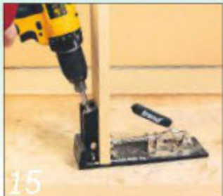
15 I used Trend's handy pocket-hole screw jig to drill all the fixing holes...
