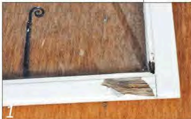
This opening casement has some rot in the bottom rail but is otherwise sound
