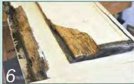
6 Both the bottom rail and two of the vertical boards were affected
