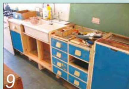
9 The kitchen gradually took shape as the various units were fitted into place
