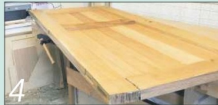
The planks had expanded across their width and badly bowed the door
