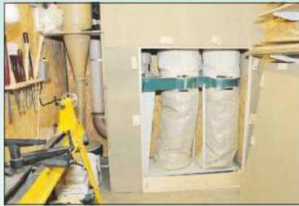
14 The Rojek extractor unit provides the suction for the cyclone unit in the corner. I moulded this myself several years ago and it works brilliantly!
