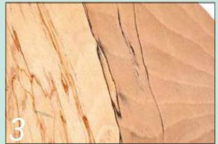
3 Problems also occur when a soft area adjoins a sound, harder one
