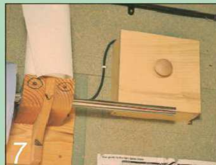
7 However, it did create quite a draught when it wasn't running, so we fit a sealed cowl over it when it's not in use
