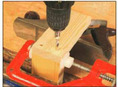
5 Drill the holes for the dowels through one component and on into the other
