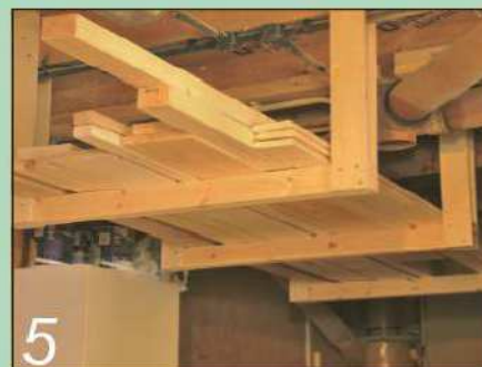
5 This rack for short-term storage will hold longer lengths of timber which we used to stack on the floor. It's connected to the joists by pairs of 12mm thick plywood hangers
