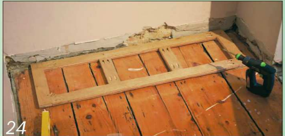
24 I set the base cabinet on a levelling frame which I shimmed with offcuts before screwing it to the floorboards
