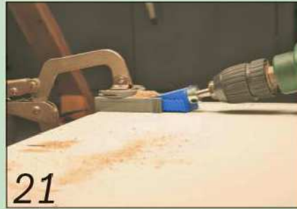
21 I drilled pocket holes in each carcass so I could attach the face frames
