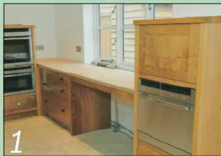
1 Under the main window we've fitted two sheets of 18mm plywood which will form the support for the stainless steel worktop
