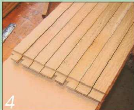
4 Cut the tenons on the ends of the eight rails, and haunch the four top ones
