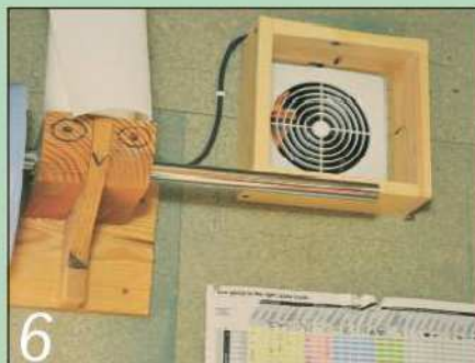
6 For our final Workshop Day job, we fitted an extractor fan in the finishing room to keep the smell of oil finishes out of the workshop
