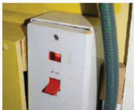
A single isolating switch which turns everything off in the workshop will give peace of mind
