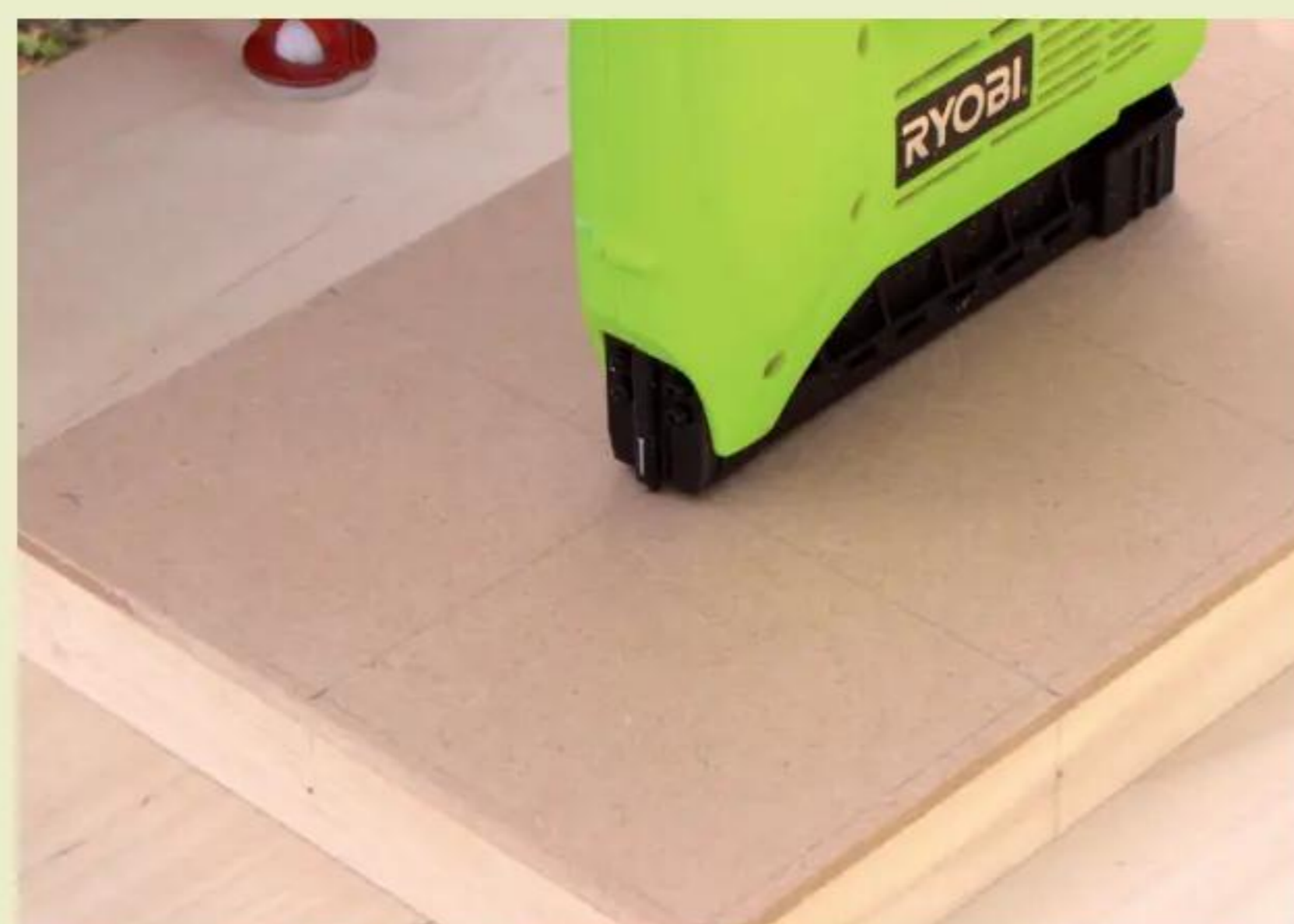
7 Position the MDF and pin to the framework, using either a nail gun or hammer and oval nails
