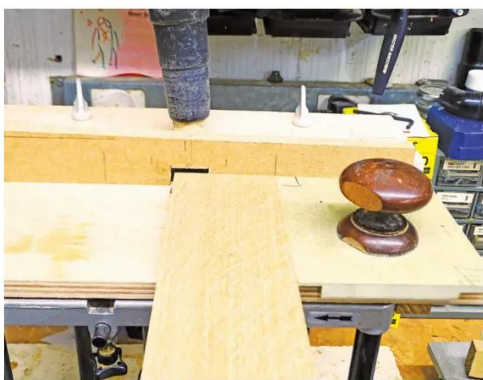
1 A scrap of MDF helps prevent any breakout when the rebate is cut
