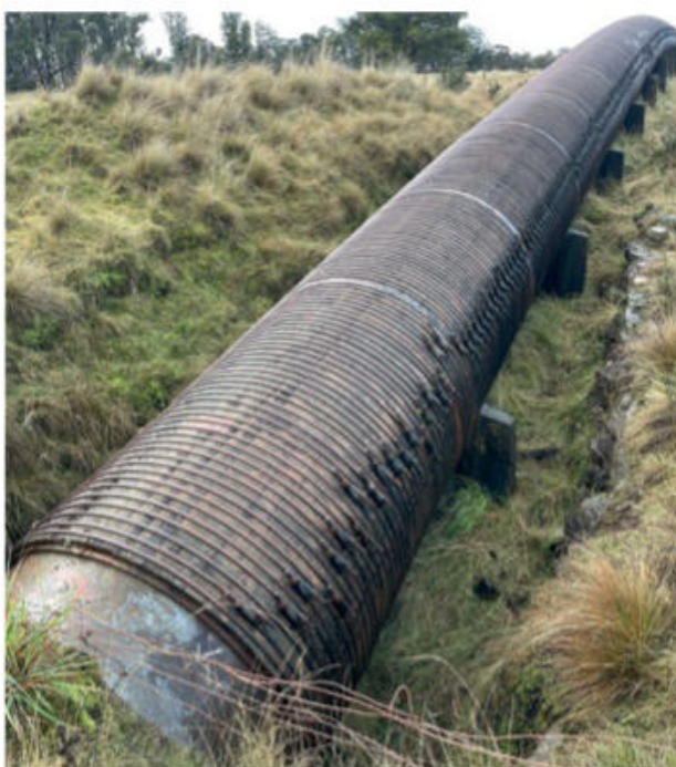
▲ This wooden penstock carries water from the Clarence river to Bronte Lagoon, Tasmania.
