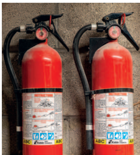
A fire extinguisher or two, of the proper type and current charge, is a low cost, very worthwhile addition to any area with wood, wood dust, and chemicals
