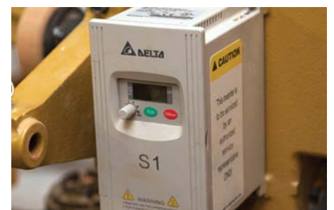
Frequency drive speed control is now inexpensive and reliable
