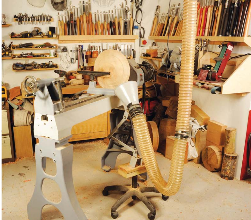
The turning area at the GMC workshop with fitted extraction ducting. It features at-source extraction via a built-in unit and ducting to each area of need
