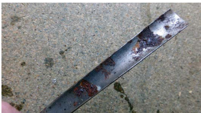
The flute suffers from localised deep rust patches
