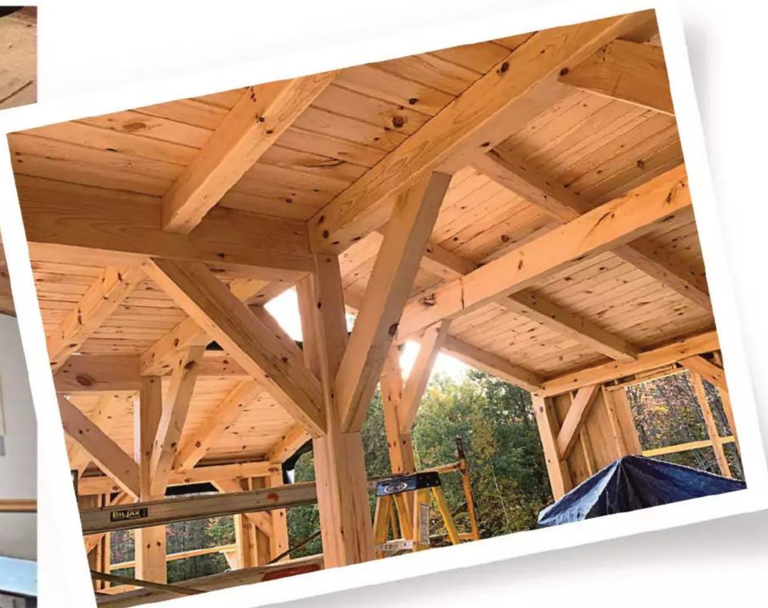
▲ Each joint in the timber frame was carefully cut and numbered to make assembly easier. Angle braces reinforce the post-and-beam connections. Tongue-and-groove sheathing encloses the roof.
