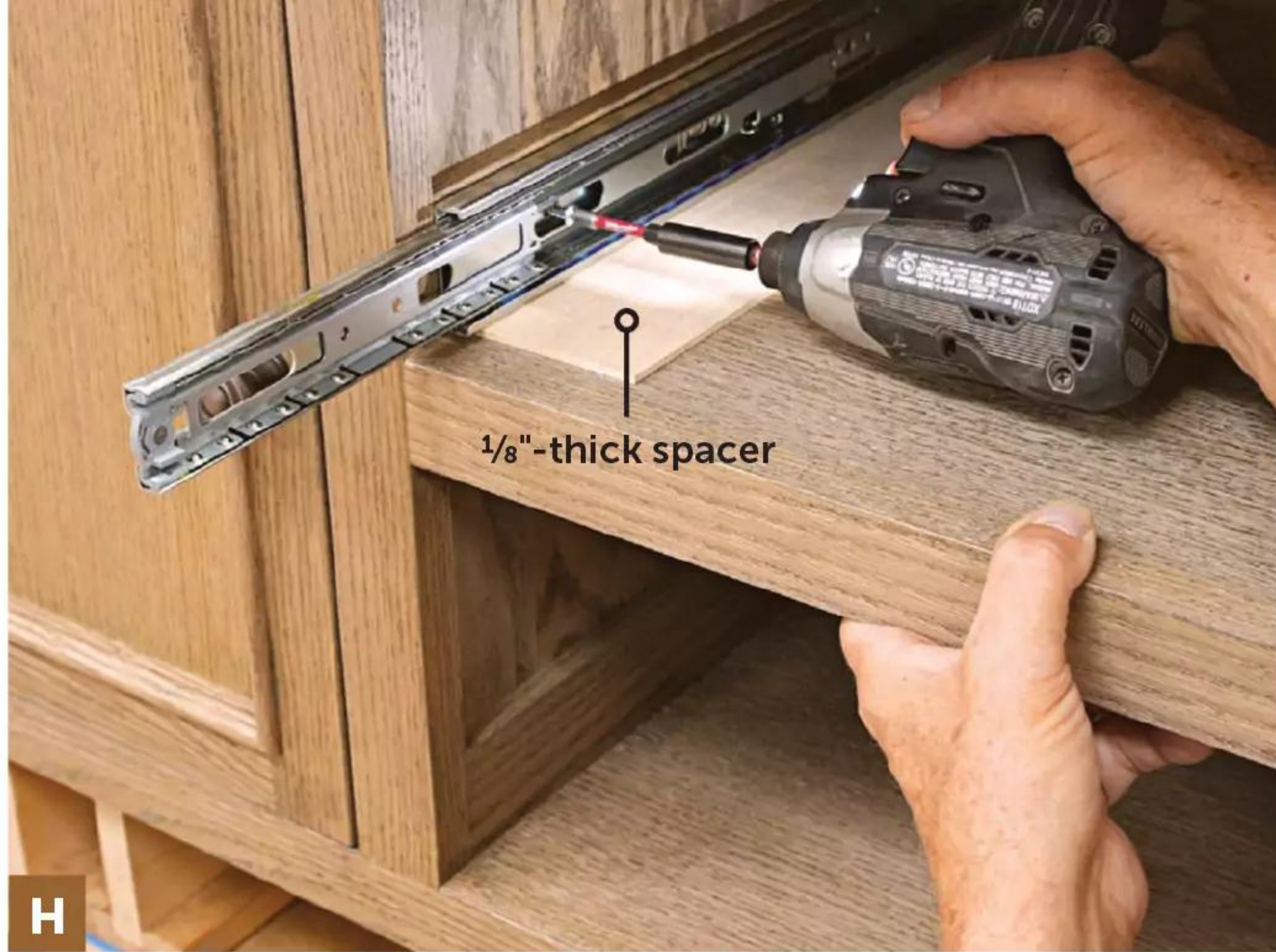
H Place a \frac{1}{8} "-thick spacer under the case portion of the drawer slide and position the front end of the slide flush with the inside edge of the face frame. Drive the mounting screws.
