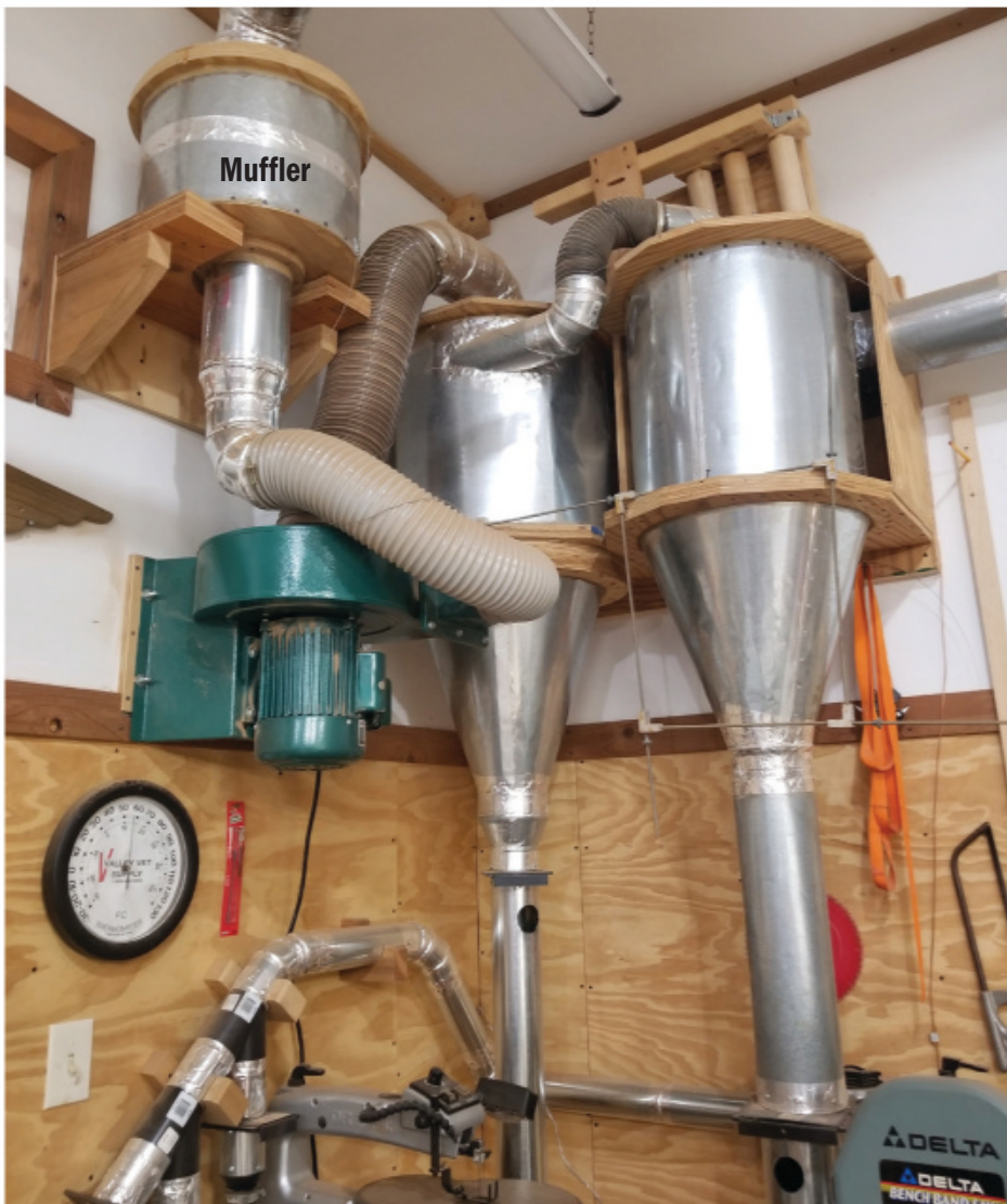
With two cyclones hooked up in series, very little dust exhausts through the roof. A shop-made muffler dampens noise during operation.
