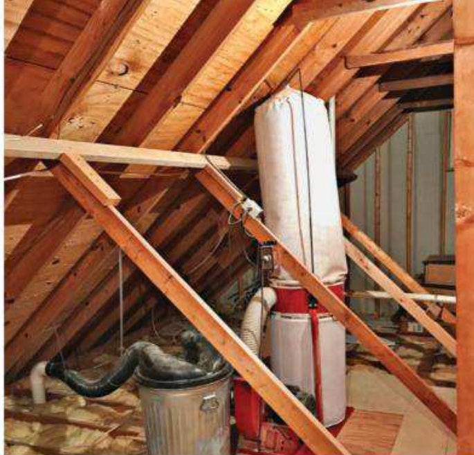
The attic houses project lumber and a dust collector with a trash-can separator. The dust collector is operated by a wireless remote control.
