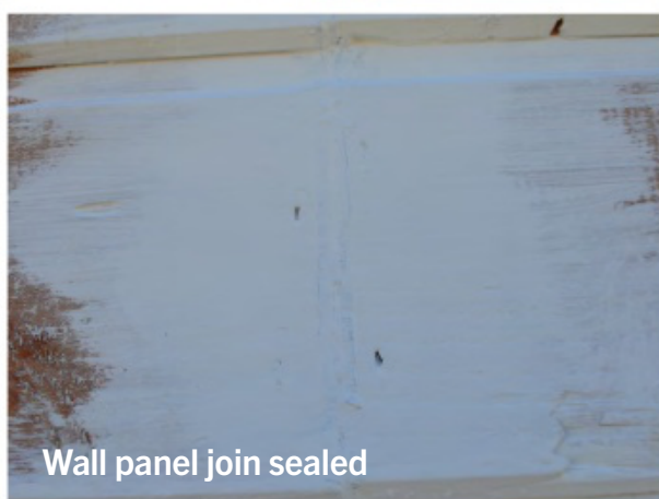
Daylight through wall panel joins
