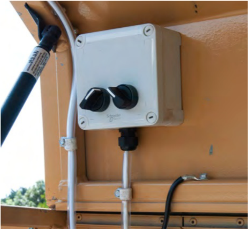
The switching for the overhead LED lighting
