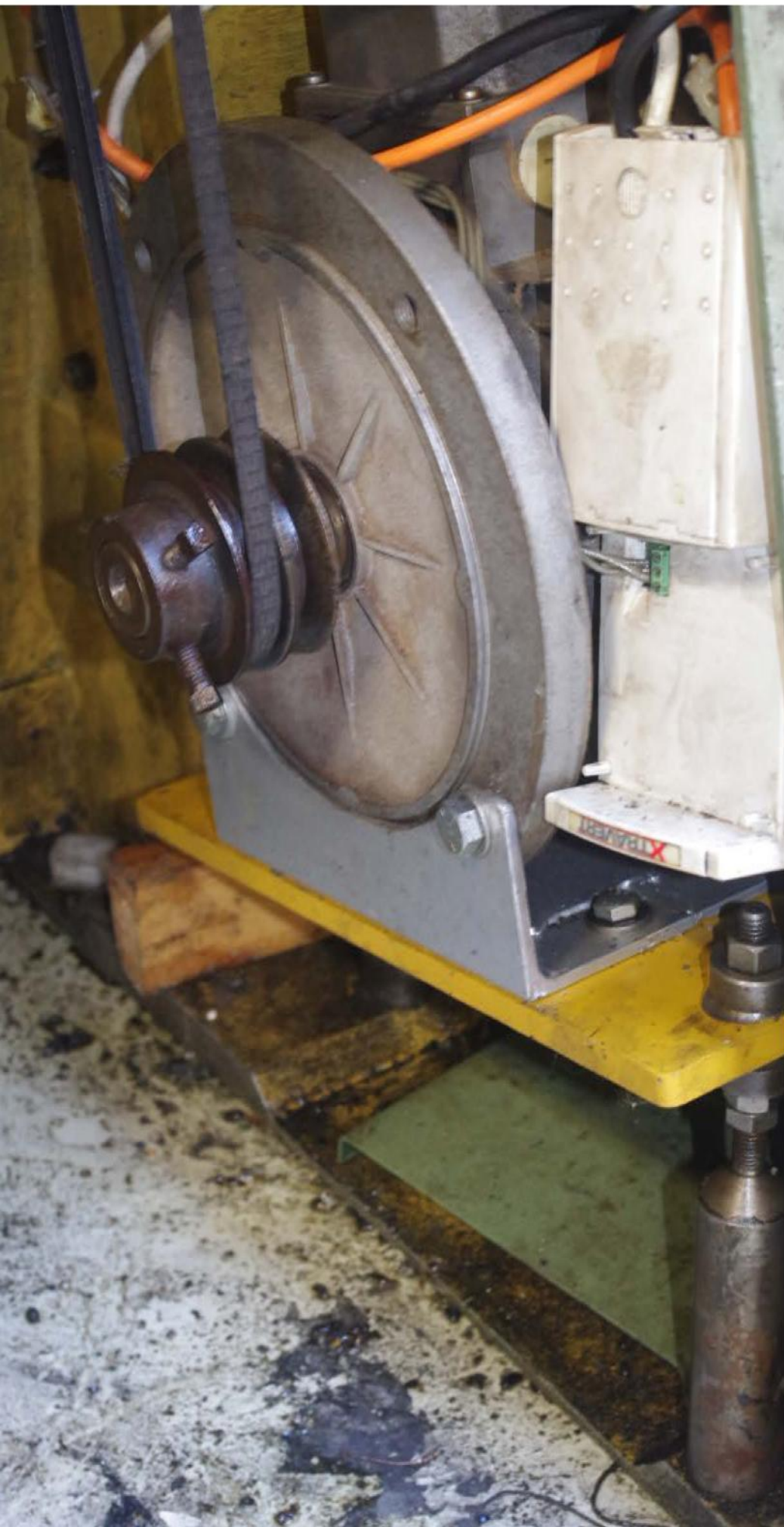
Left: VFD in base of Colchester Chipmaster. Yes, the drive is upside down — not recommended for cooling, but it has been on the list to change for the past five years since I changed the motor over
