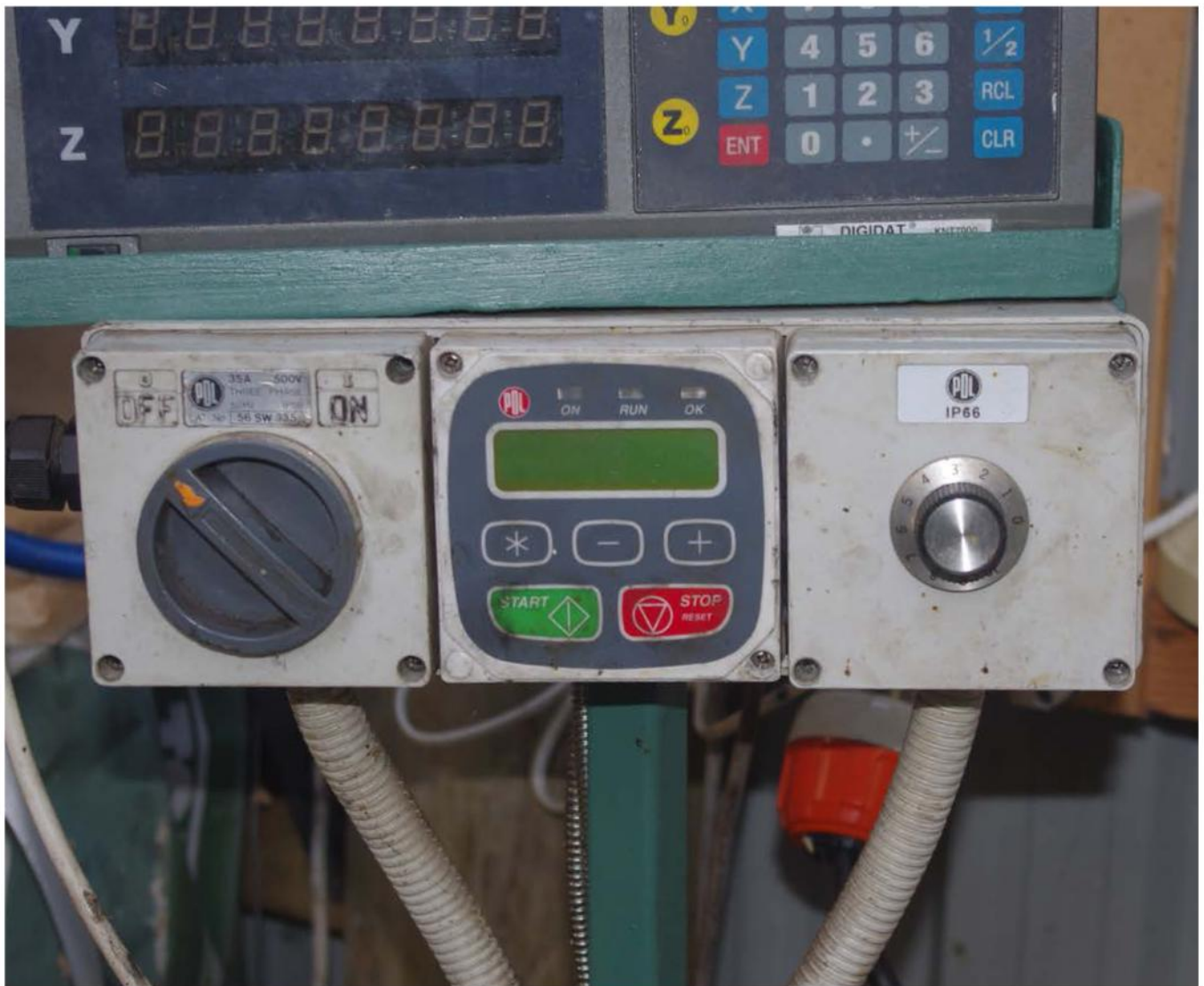
VFD remote-control panel with speed adjustment knob
