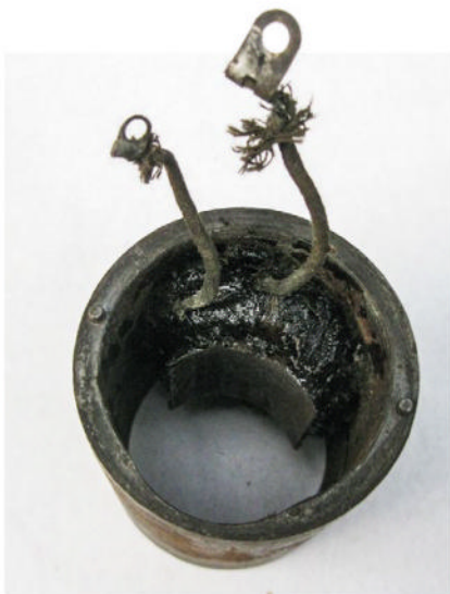
The generator case with its field coil, but the rest of the innards have been removed
