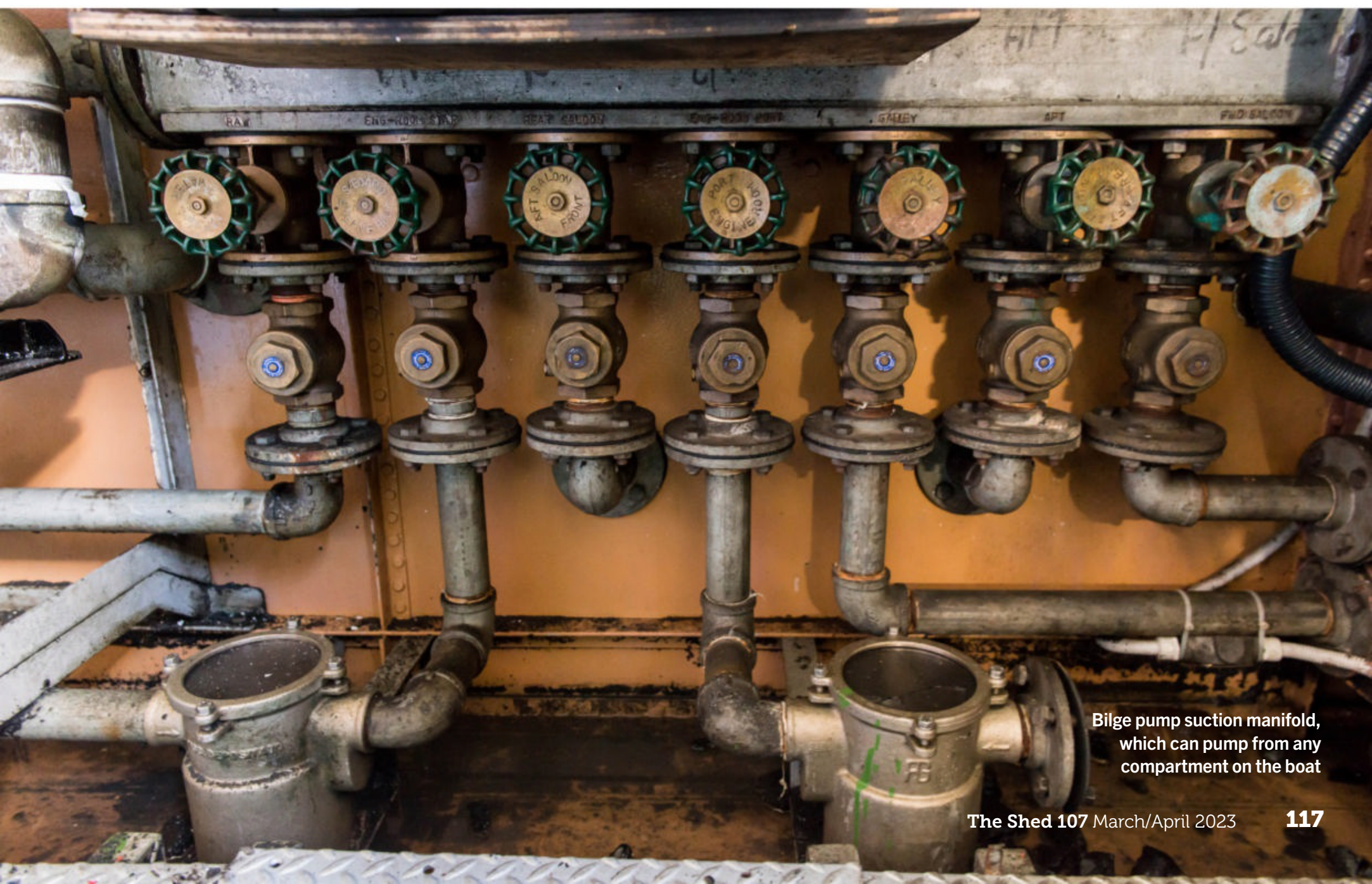
Bilge pump set-up: steam pump above, hand pump below
