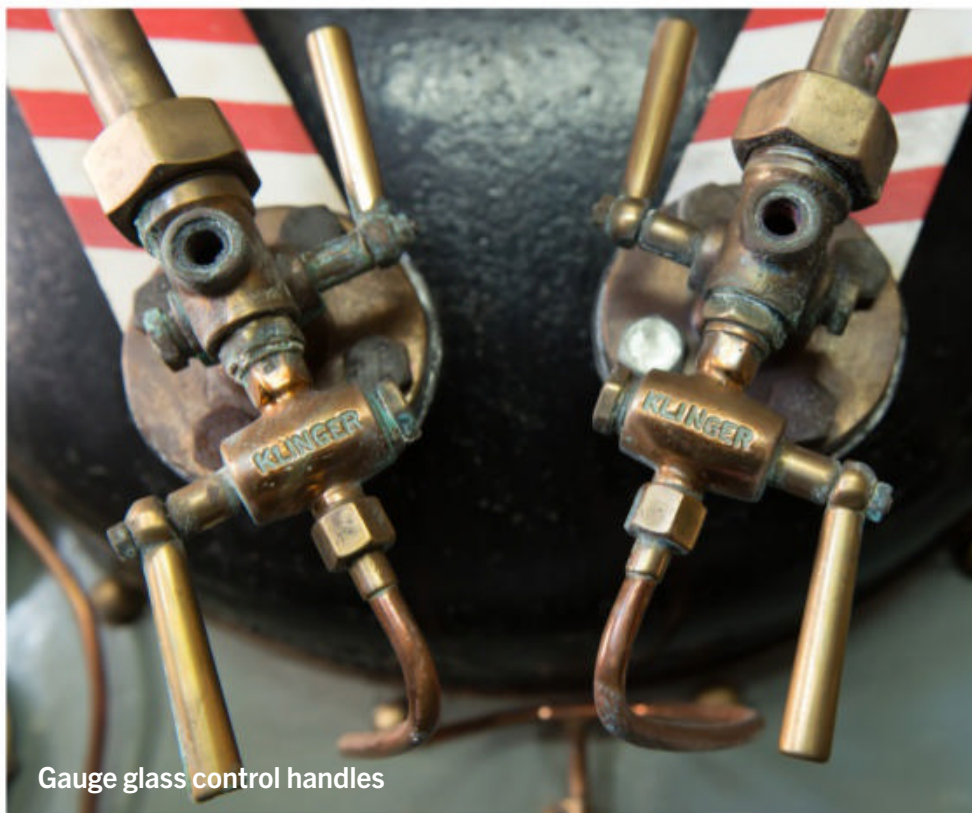
Steam valve bonnets ready for inspection
