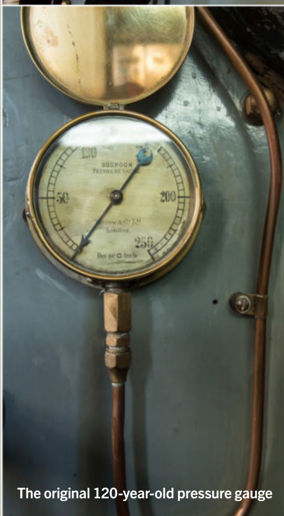
The boiler stripped down for its annual survey
