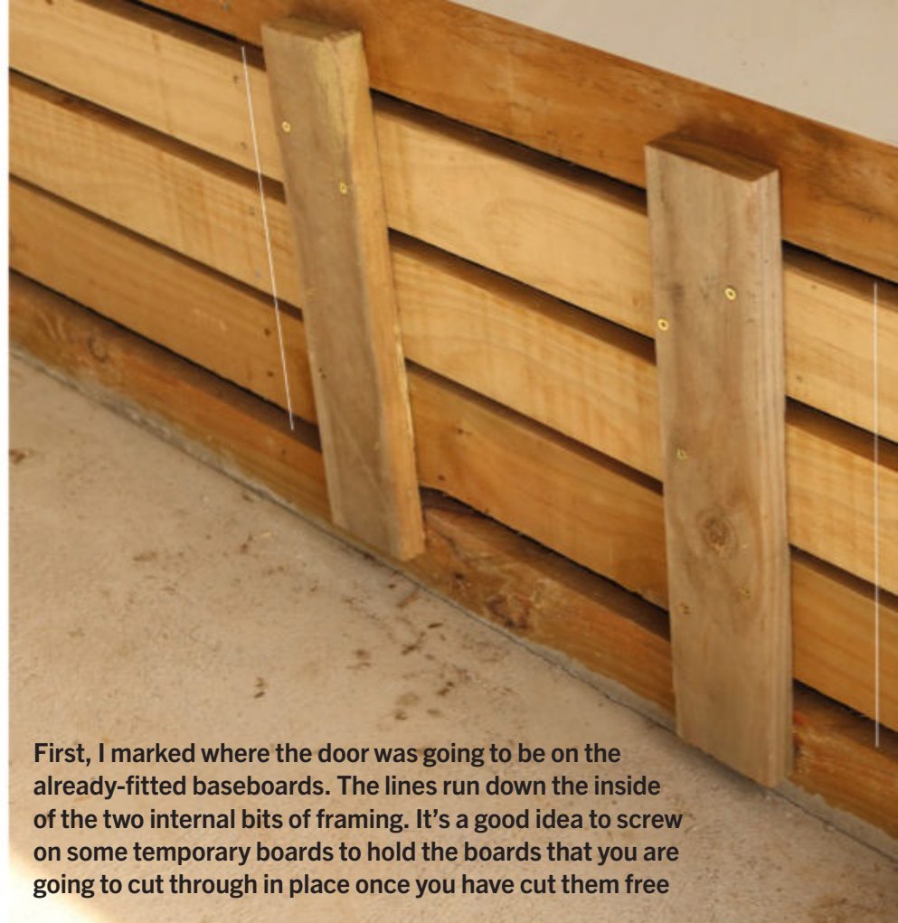
The completed section of the baseboards, but no way to get to the water valve
