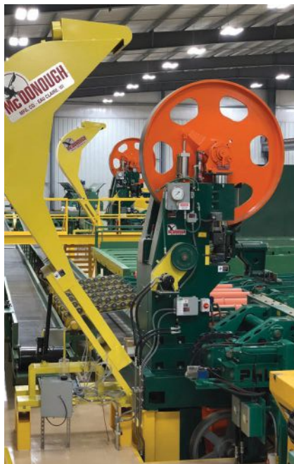
Two new McDonough resaws were installed at the new Emporium Hardwoods mill in Emporium, PA.
