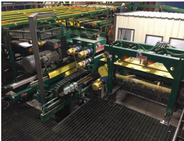
Pictured is McDonough's new Curve Sawing Gang installed at High Country Lumber and Mulch in North Wilkesboro, NC.
