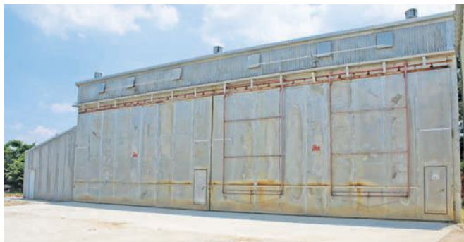
Two dry kilns by SII Dry Kilns are pictured that hold 50,000 board feet each and are located at R&M Wood's property. The company dries 300,000 board feet of lumber monthly.
