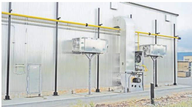
Thompson Appalachian Hardwoods in Huntland, TN has two 100,500 BF Package Kilns with Heat Exchangers and Direct Fire Burner.
