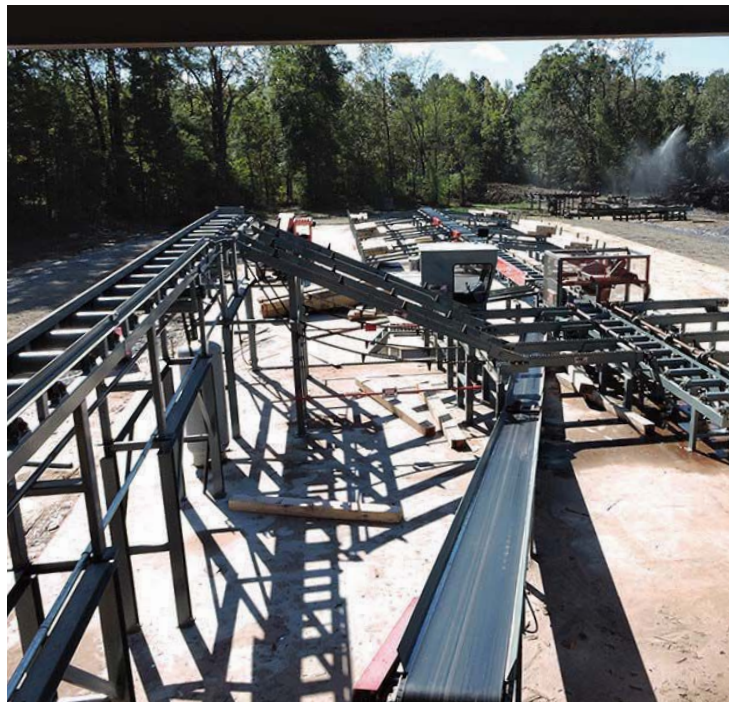
This is Fred Netterville Lumber's new American Built Machinery timber processing line.
