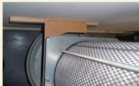
19—Bracket holding filter assembly to the wall
