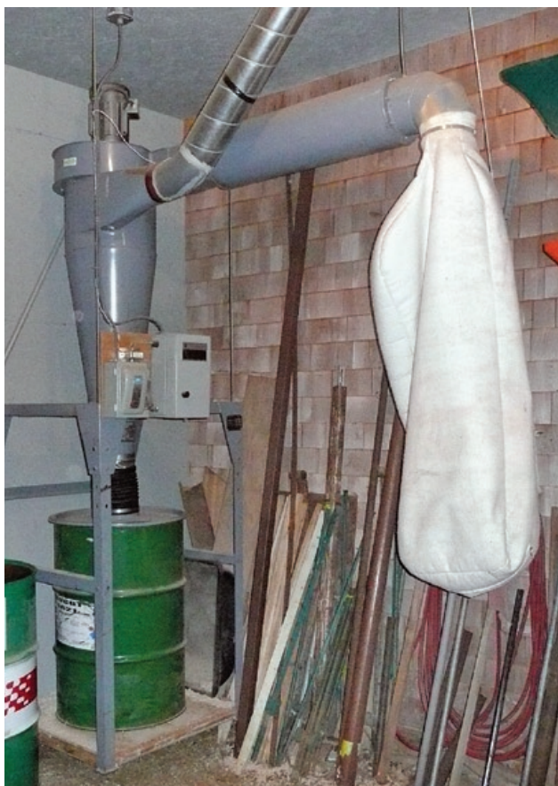
1—This is how the system looked before I started
