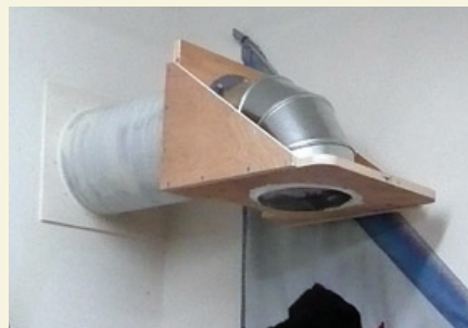
13—Support bracket mounted to end of sound dampener
