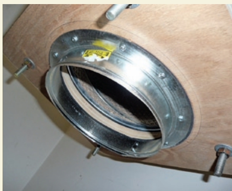
20—Flange at bottom of filter assembly
