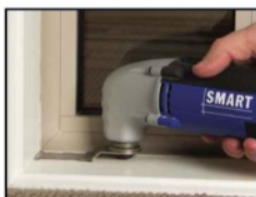
UNDER CUTTING DOOR JAMBS
