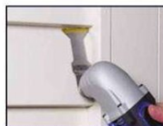
UNDER CUTTING WEATHER BOARD
