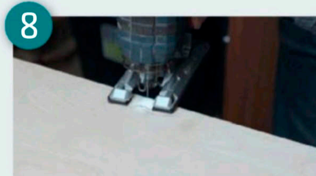
At the back is a semi-circle to route all the cables through
