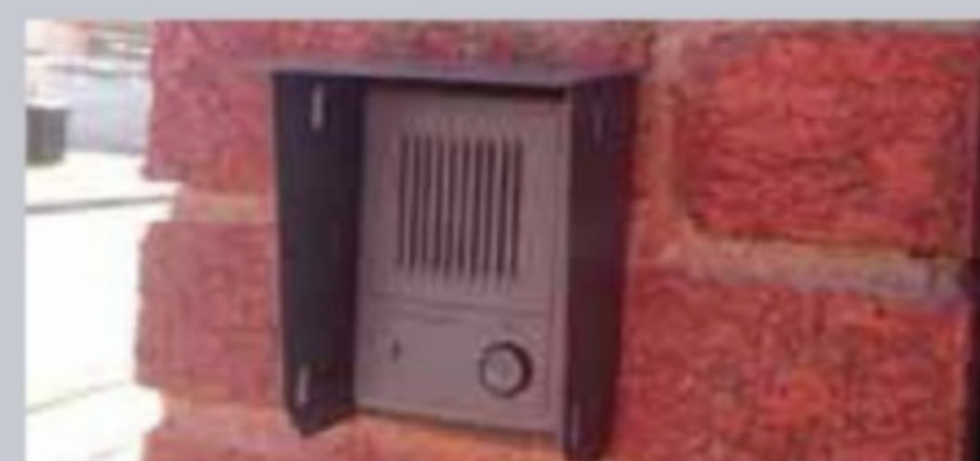
A gate intercom can be a convenient method of communication to visitors but can also be subject to vandalism. In today's world of mobile phones, intercom systems should be confined to offices
