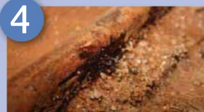
The corroded water pipe
