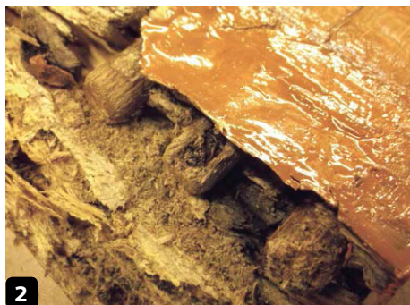
2 Close-up of a rotted joint
