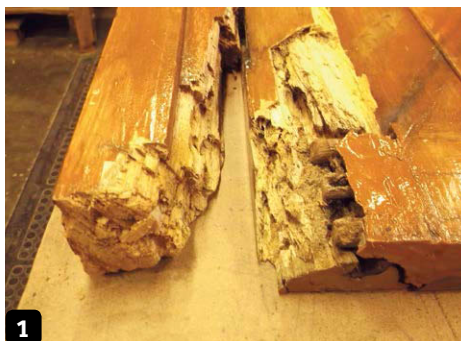
1 Rot beyond repair
