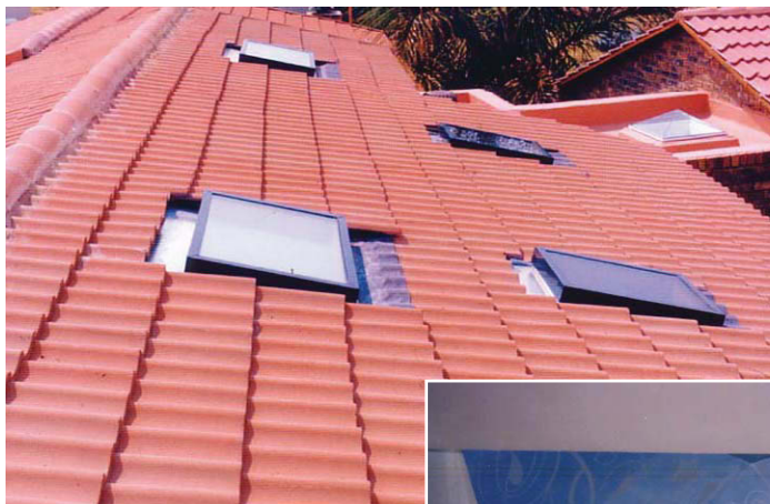
Skylights successfully allow in light on south-facing roofs
