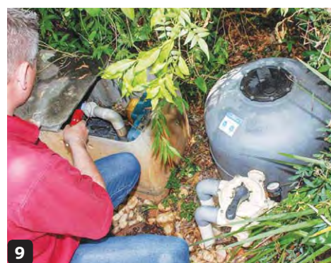
9 Secure the lid on the tank again and set the pump valve to the 'filter' cycle
