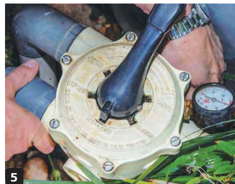
5 Set the pump valve to 'backwash' for five minutes
