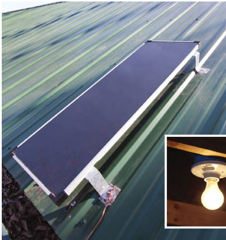
A solar panel connected to a battery-powered lighting system can provide plenty of light to remote buildings or sheds.
