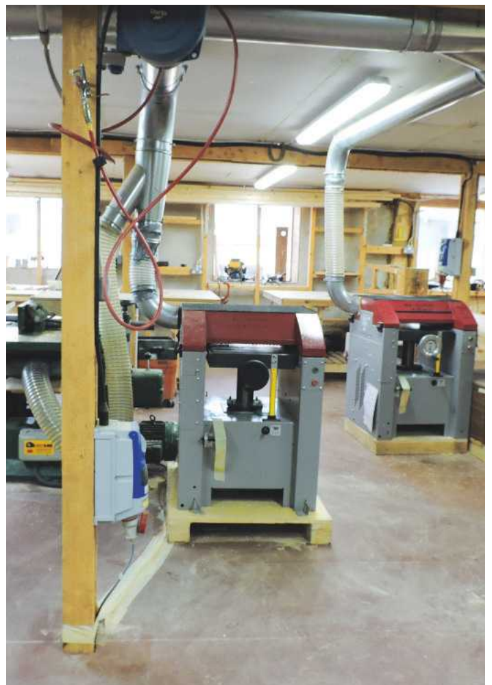
One of the school's well equipped machine shops
