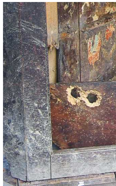
This damage has destroyed the core strength
