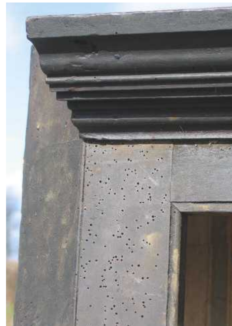
Typical woodworm damage
